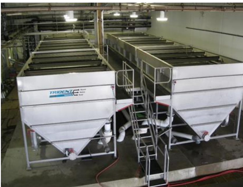
Two 400ft 2 DAF tanks float the nutrients where they can be skimmed off and converted into dry, stackable fertilizer.
