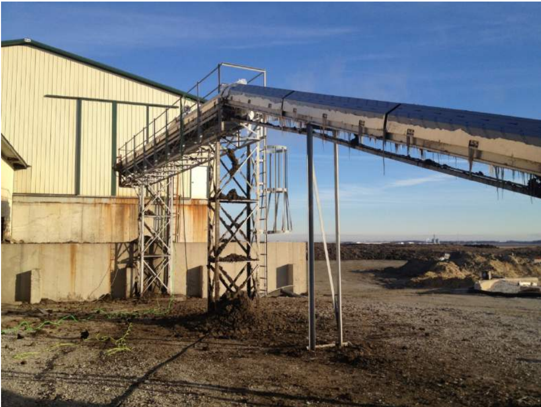
10 Solids transfer conveyor
