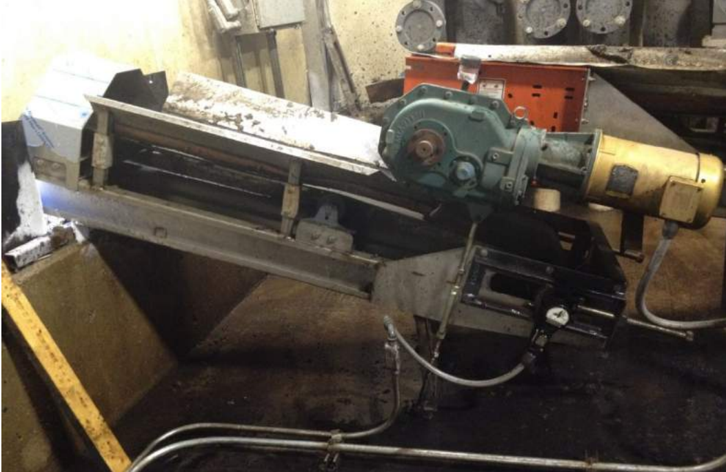
9 Solids discharge conveyor
