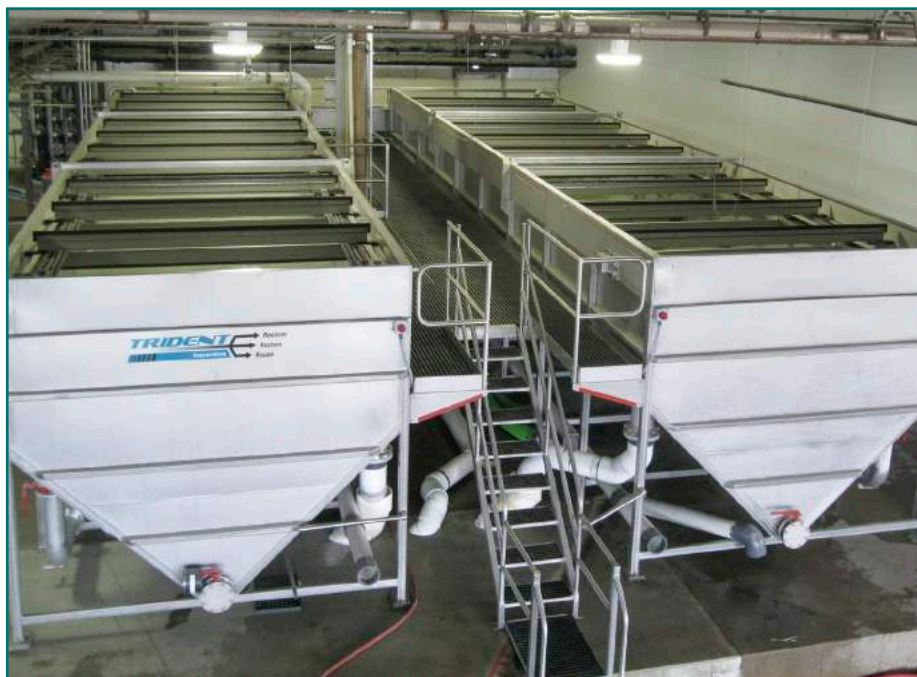
Two 400 sqft DAF tanks at a 14,000 cow site with anaerobic digester.
