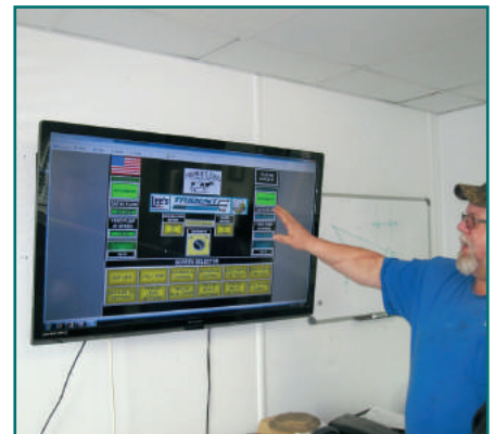
The automation system gives operators access to real-time data.
